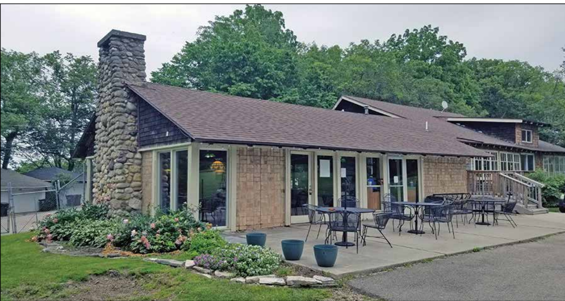
Work is underway at the Lauderdale Lakes Country Club, where the old clubhouse and patio are being torn down to construct new ones from scratch. This picture shows the old clubhouse and patio.
