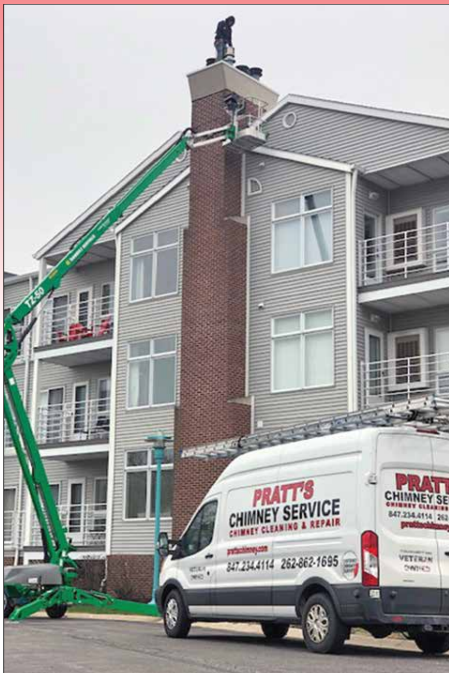
A technician from Pratt's Chimney Service works on the chimney to be certain it is safe for use.
