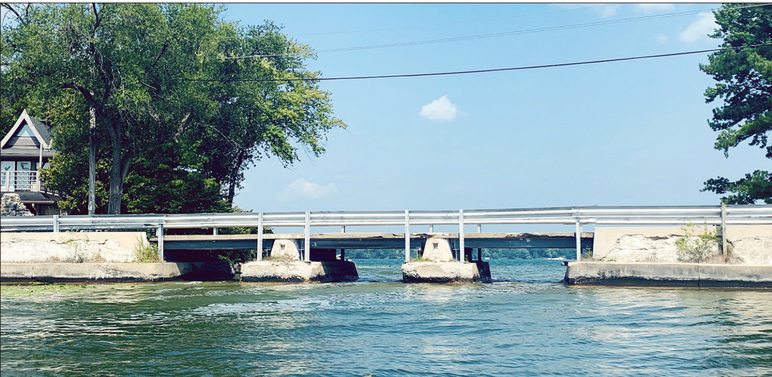
The Lauderdale Drive Bridge, also known as the Deakin Isle Bridge, which goes over Green Lake in the Town of La Grange, is scheduled to be replaced this fall.
