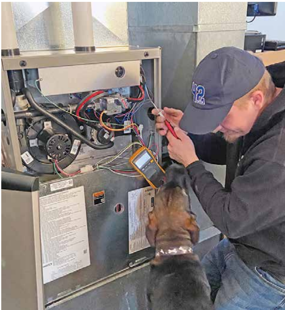
Technician Nick Romani services a furnace. Each furnace should be serviced yearly before the heating season begins to assure that it works properly throughout the season, he said. In spring the air conditioner needs to be serviced.
